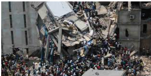
Fig. 3: Picture of the Rana Plaza in the aftermath of the building collapse. Source
